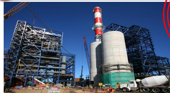
Coal fired plant, 350 MW
